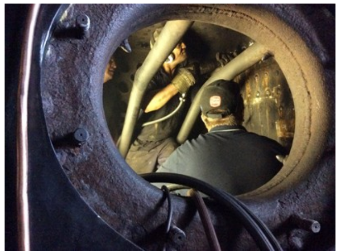
Inside the firebox
